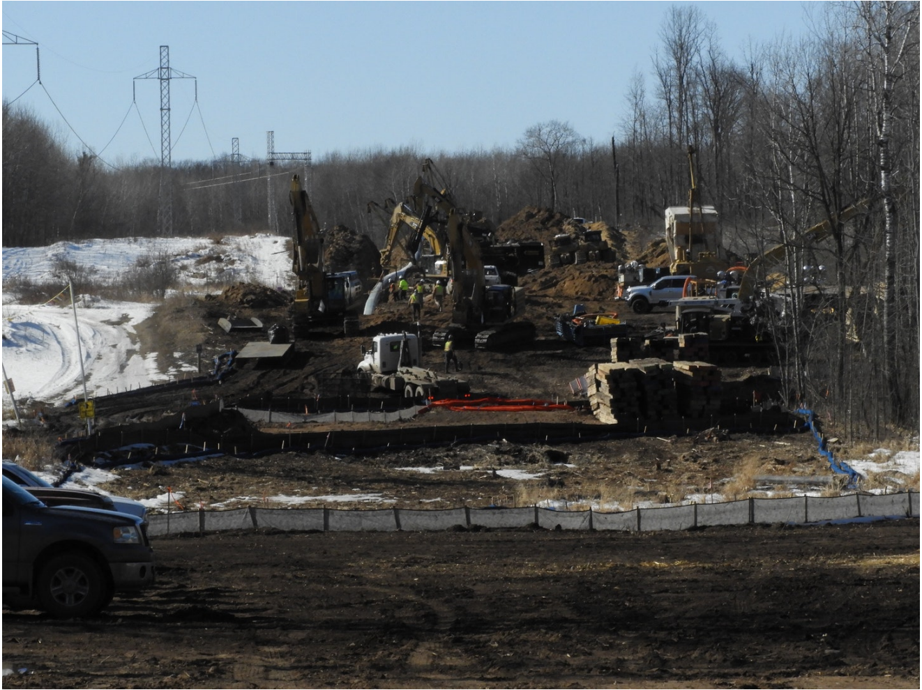
That same spot in Cass County, Minnesota, just east of the Moose River, after Enbridge started construction on Line 3. Photo: Aimee Sutherland.
